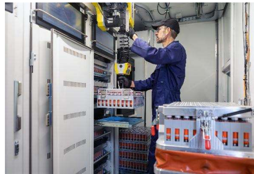
Figure 2: Nodal system camp operations using a motorized lifter to batch-handle 90 nodes into a high capacity charging/download rack.
